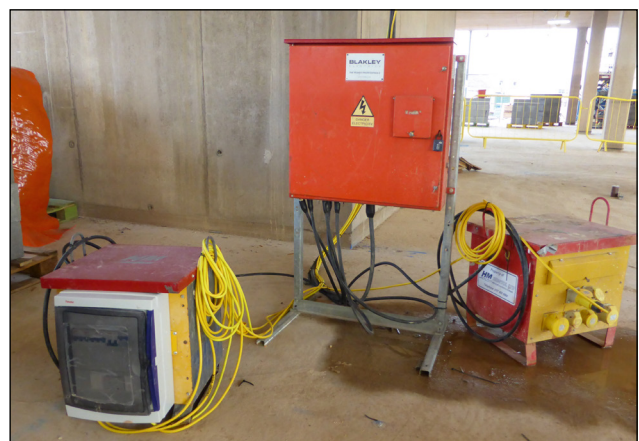
Figure 5 Examples of temporary distribution equipment appropriate for a construction site
