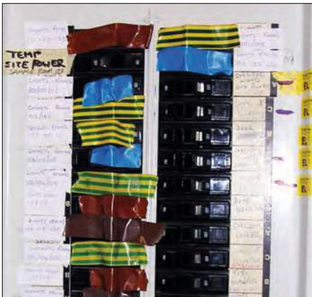
Figure 4a An example of bad practice – tape covering circuit breaker
