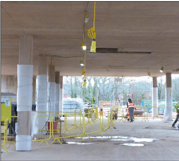
Figure 6 Cabling fixed at height eliminating the need for extension leads and trailing cables
