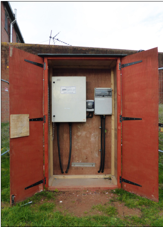
Figure 1 Main site intake point for a new-build construction site
