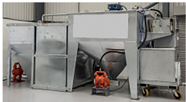
Figure 15 Waste water/slurry management system
