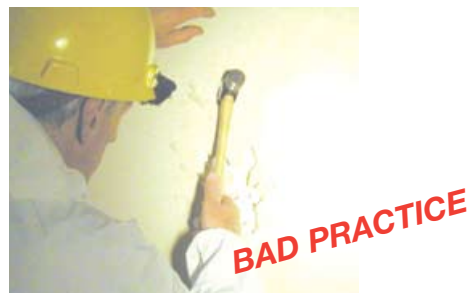
Figure 5 Maintenance worker, working on asbestos insulating board without adequate controls
