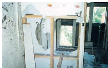
Figure 7 Asbestos insulating board wall panels badly damaged
