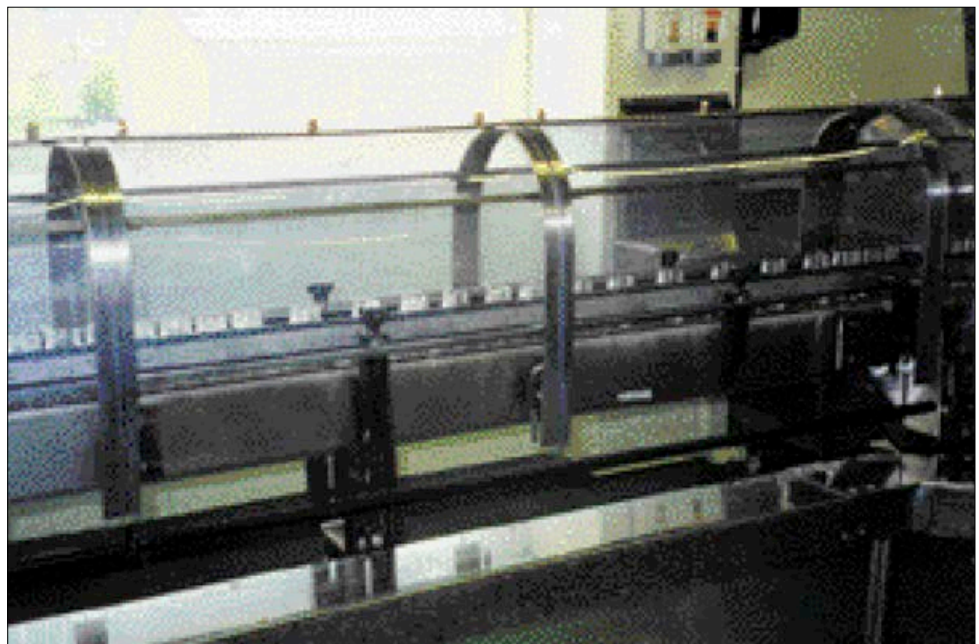
Problem: enclosure over glass jar conveyor
