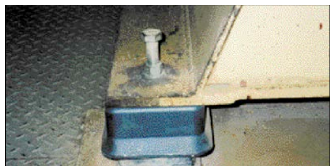
Solution: close-up of anti-vibration mount
