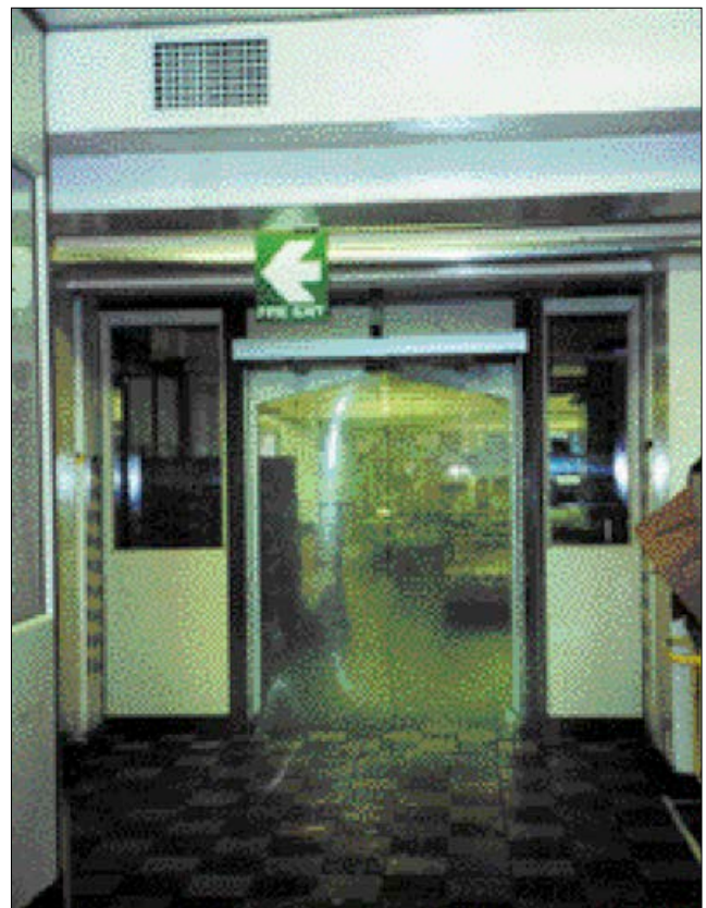
Solution: automatic, flexible PVC curtain doors installed to segregate ear protection zone from quieter area
