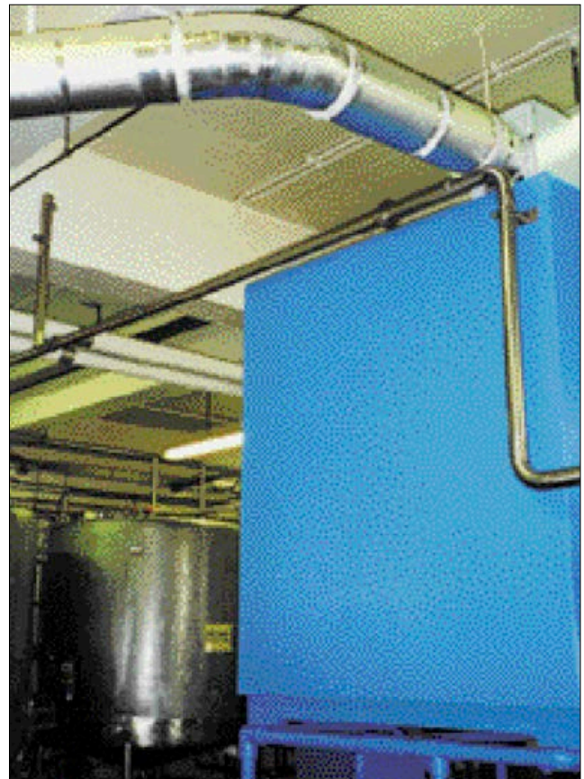
Solution: transport ductwork (top of photo) lagged externally with noise-absorbent padding
