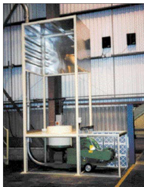
Solution: new blower machine installed in enclosure (sound-absorbent side panels removed for clarity)
