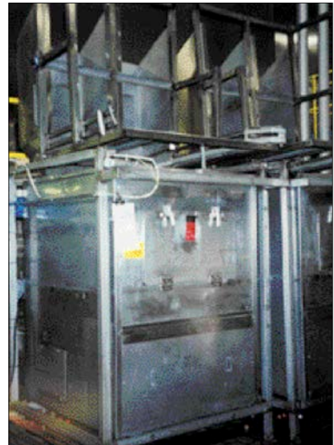
Solution: stainless-steel cap-hoppers inside new segregated enclosure
