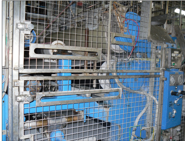
Figure 28 Press section enclosed with fixed guarding
