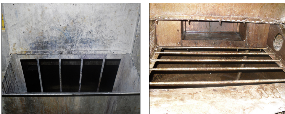
Figure 20 Example of fixed grilles on side and top openings of a pulper. Both fixed grilles have been added to prevent whole body access
