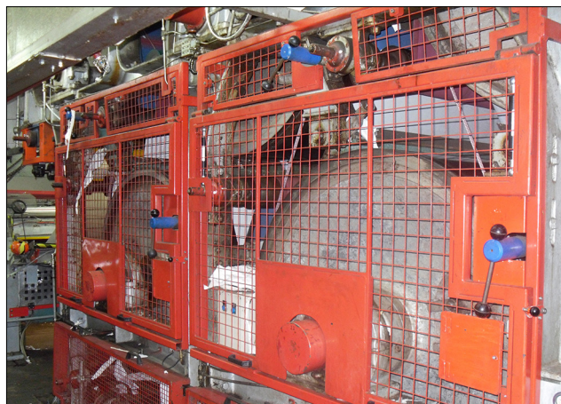
Figure 2 Example of fixed guarding in place to prevent access to the drying cylinders on a paper machine
