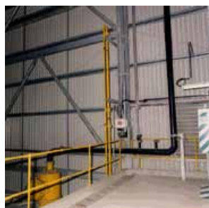
Lute pipe (barometric leg) and vent for absorption system
