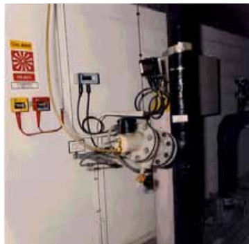
Chlorine detector alarm in vent line from absorber
